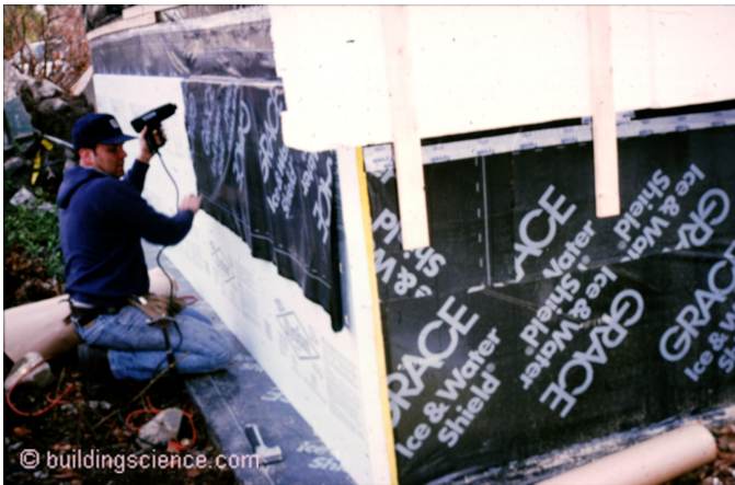
Photograph 3: Aluminum Sheet – Rigid insulation with a membrane seal prior to installation of the aluminum.
