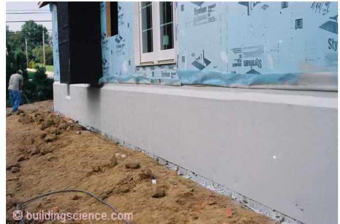
Photograph 1: Stucco as Protection - It has impact limitations, but it actually looks very good.
